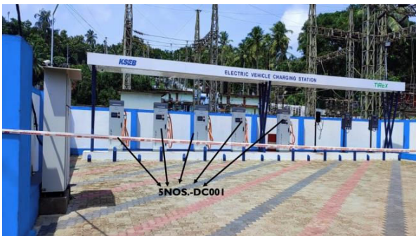
DC Fast charging stations.
