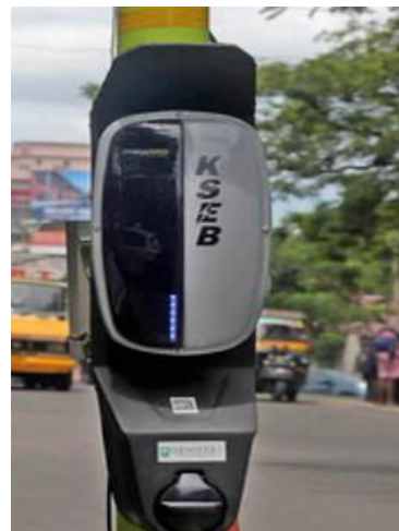
Pole mounted EV charging stations
